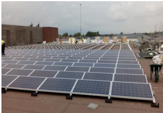
Solar PV panels at Northgate Arena, Chester
