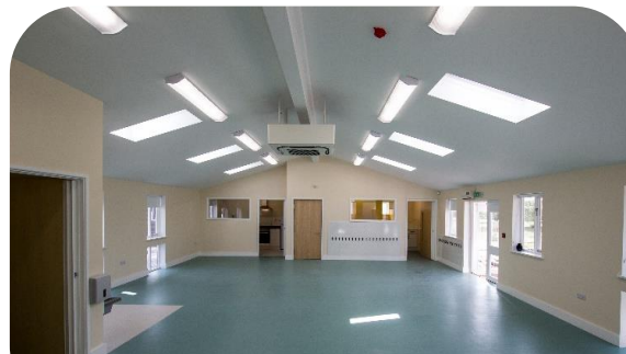
Guilden Sutton Village Hall LED retrofit
